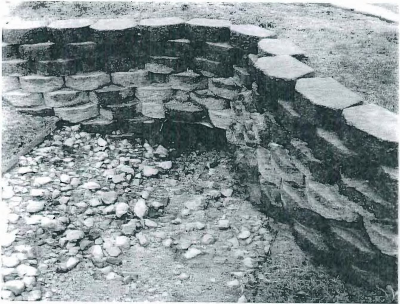
Photo 14 – Next culvert, filling with deposits
