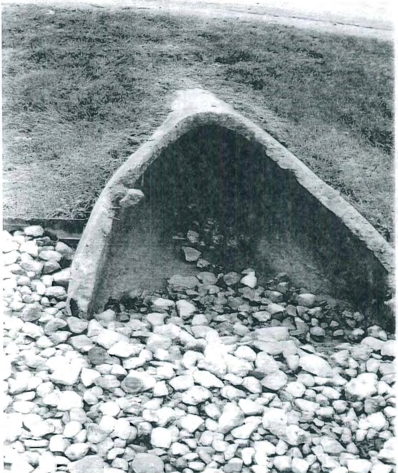
Photo 7 – Culvert exit on north side of road. Note the deposits on the pipe wall and rocks that are the same color as the wash water in the basin.
