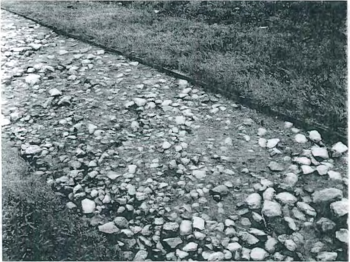
Photo 8 – Road ditch on north side of street with deposits on rocks.
