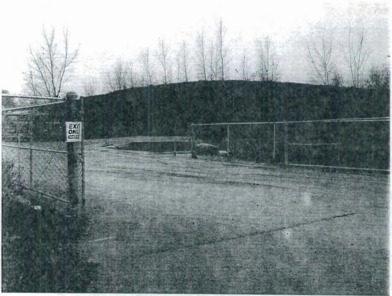
Photo 18 – Concrete truck wash out area on northeast corner of property near facility exit.
