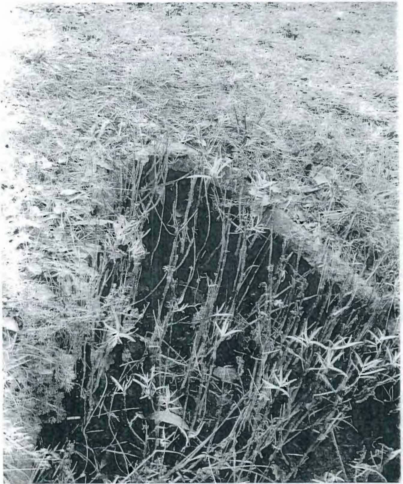
Photo 6 – Flow enters the culvert at this point and goes north under the road. Note deposits in culvert that are the same color as the wash water in the settling basin.
