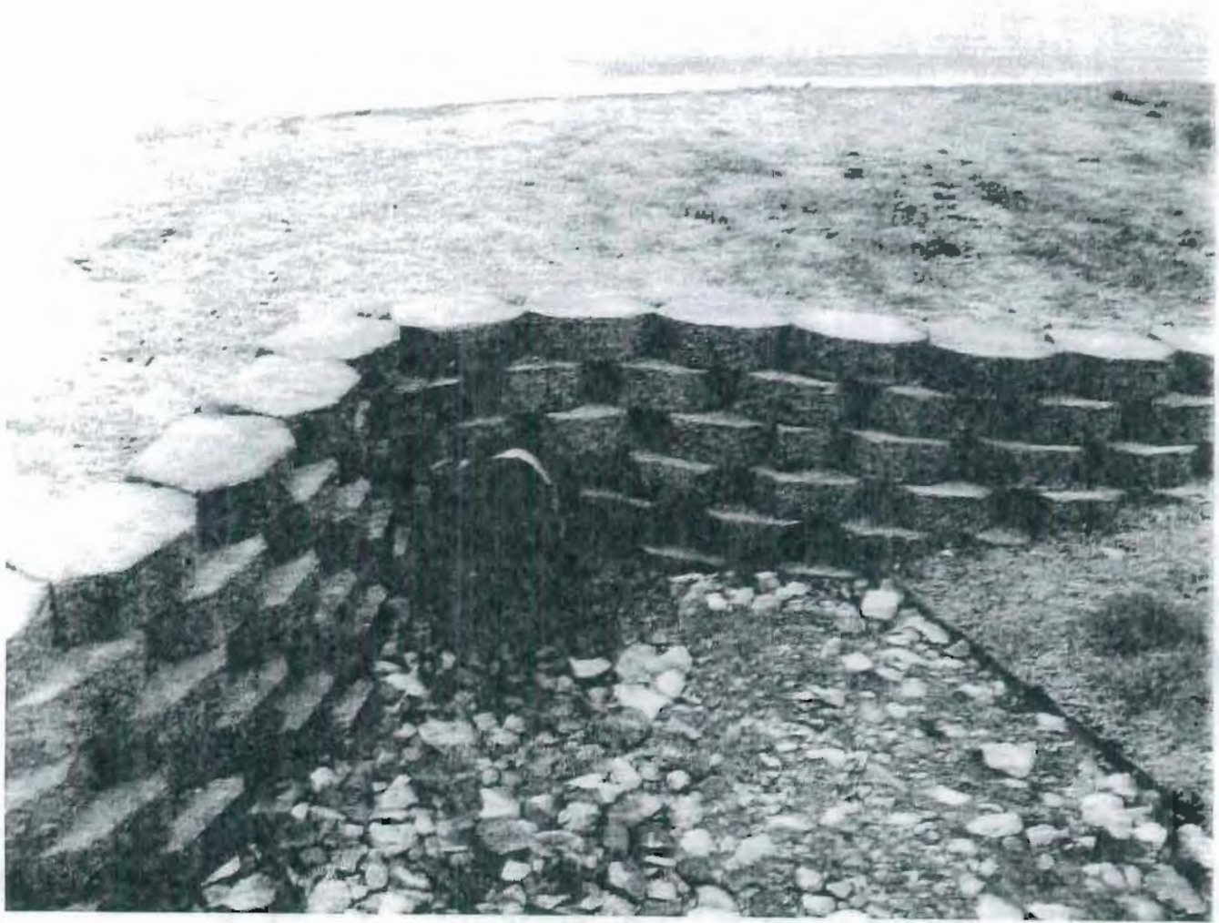
Photo 9 – Flow path continuing east showing deposits entering culvert under driveway
