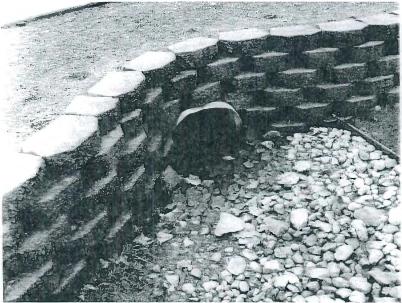
Photo 11 – Culvert exit on other side of driveway showing murky water and deposits on stones
