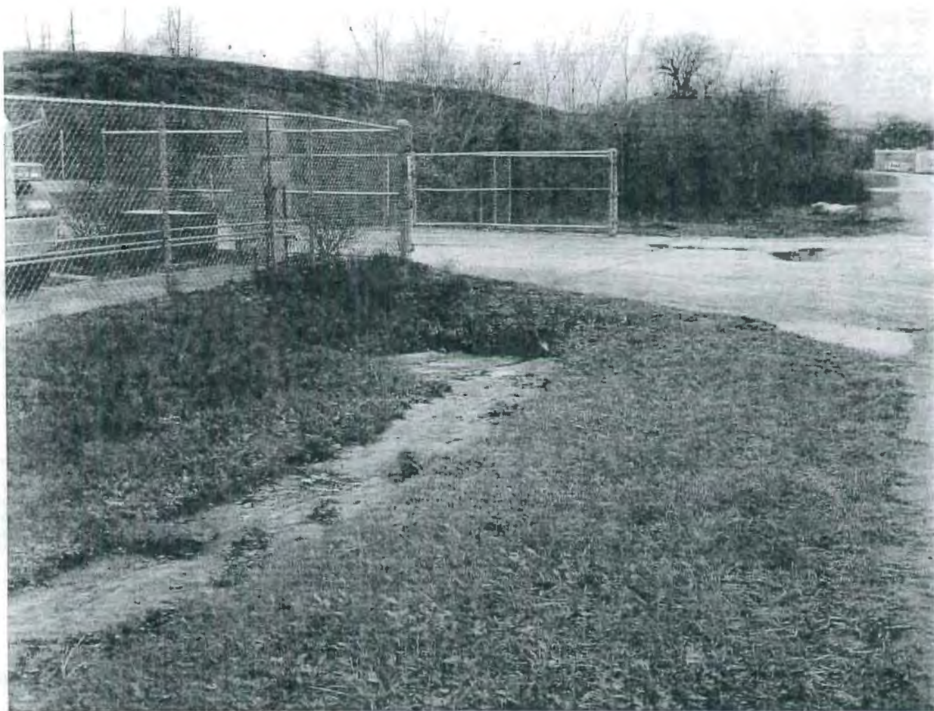
Photo 17 – Following road ditch west, showing another discharge point and the deposits in the ditch.
