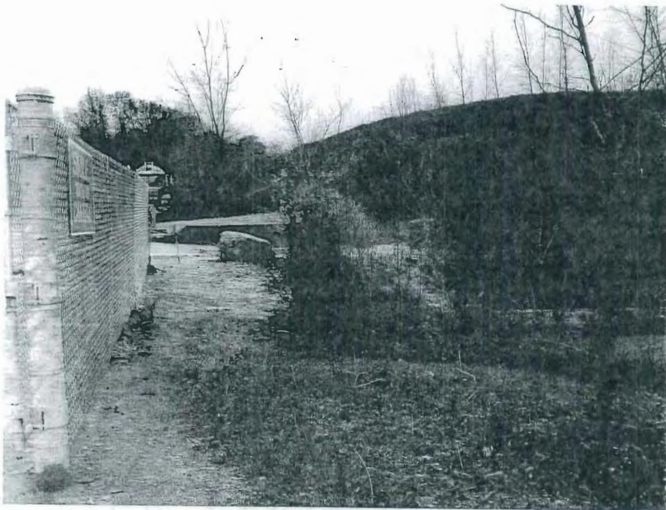
Photo 19 – shows how flow is able to run off the property from the wash area into the settling basin in the road ditch.
